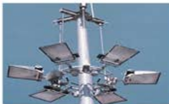
High Mast Lighting
